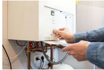
A man lowers the temperature on a gas boiler (Image: Getty)
